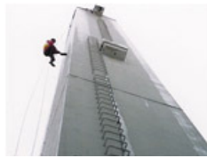
Craven Black Cat Tower Hammer Test and Visual Survey to high rise concrete Art Deco Chimney.
